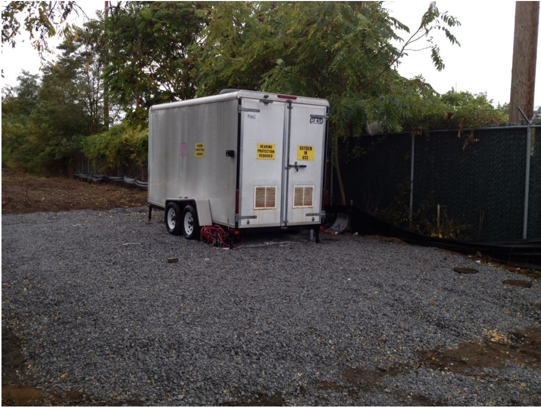
Relocated 60/66 North Clinton Avenue oxygen injection system
